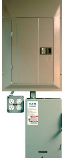
MAIN SERVICE PANEL MASTER CUT-OFF SWITCH & UTILITY OUTLET
